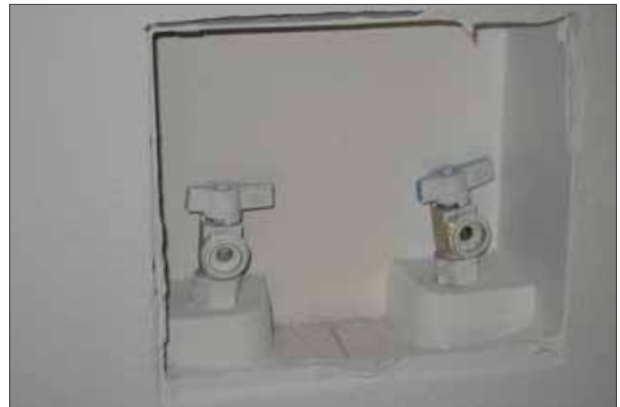
Unprotected Opening. Open boxes are susceptible to drywall mud, paint, dirt and debris or require added time and material to protect them.
