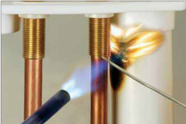
Crowded Lines. Close proximity of drain and supply lines can require extra fittings or lead to damaged fittings/pipe from glue or flame.
