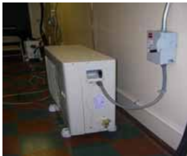
Local Disconnect and Whip Connected
