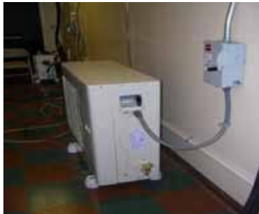
Local Disconnect and Whip Connected
