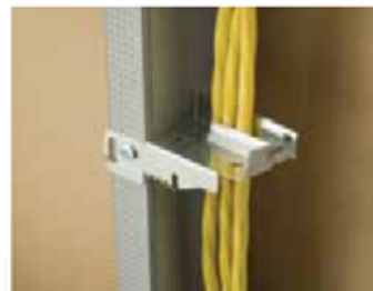
Metal Stud with non-metallic sheathed cables
