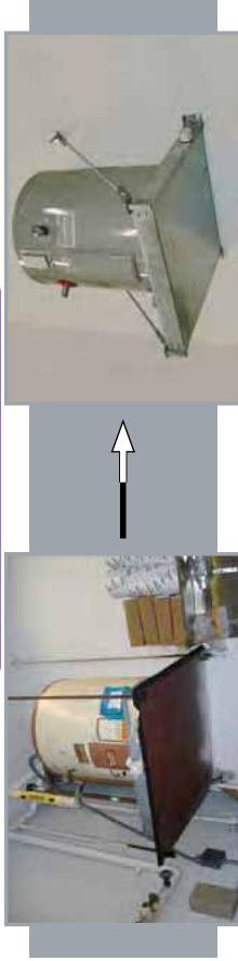
WATER HEATER SUPPORT
